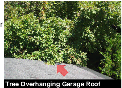
Tree Overhanging Garage Roof
